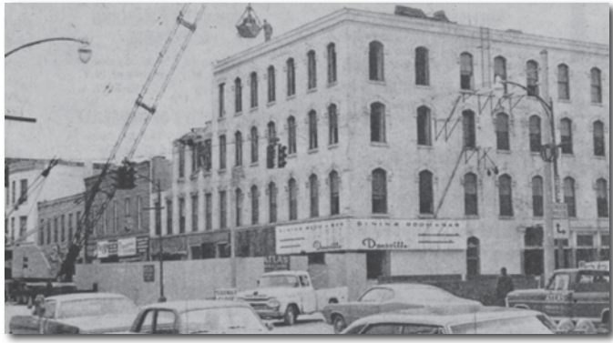
On April 5, 1971, demolition was beginning on the Hotel Dansville. Just below the man and bucket, and also behind the fire escape, the name "Hyland" was still visible, denoting the original owners. Today, the Community Bank building occupies that corner. (Photo by Wilfred J. Rauber)
