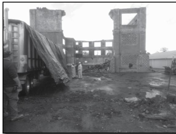
Photo taken February 21, 2014, showing demolition of the Blum Shoe Manufacturing Company building. HazMat suits are being worn by asbestos abatement workers as they truck away interior material from the building. This photo was taken looking north towards Milton Street.
